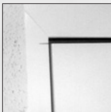
5. The gap at the top left corner of the doorframe.
